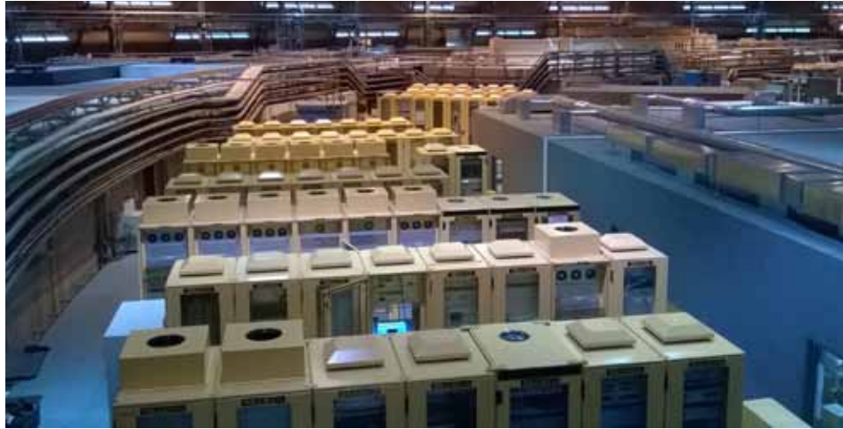
A partial overhead view of the storage ring and support equipment of SLS. Photo: Nikolaos Papakonstantinou.
