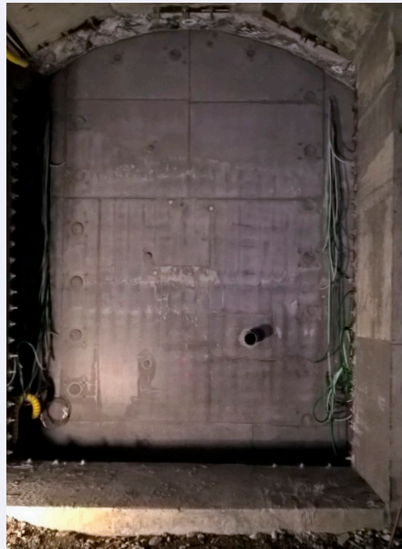
Figure 4. The final cast plug, 6 metres in height at 420 metres underground at ONKALO, within the DOPAS project. (Photo: Erika Holt)
