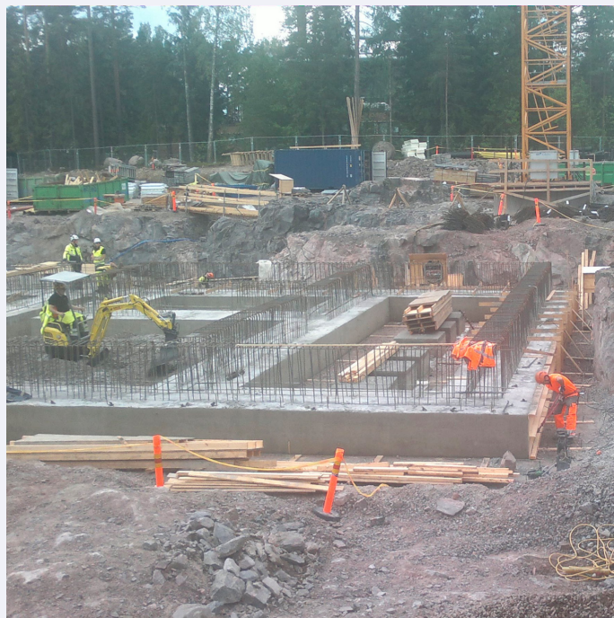
Figure 1. Six months after site preparations began in January 2014, the massive footings were ready.
