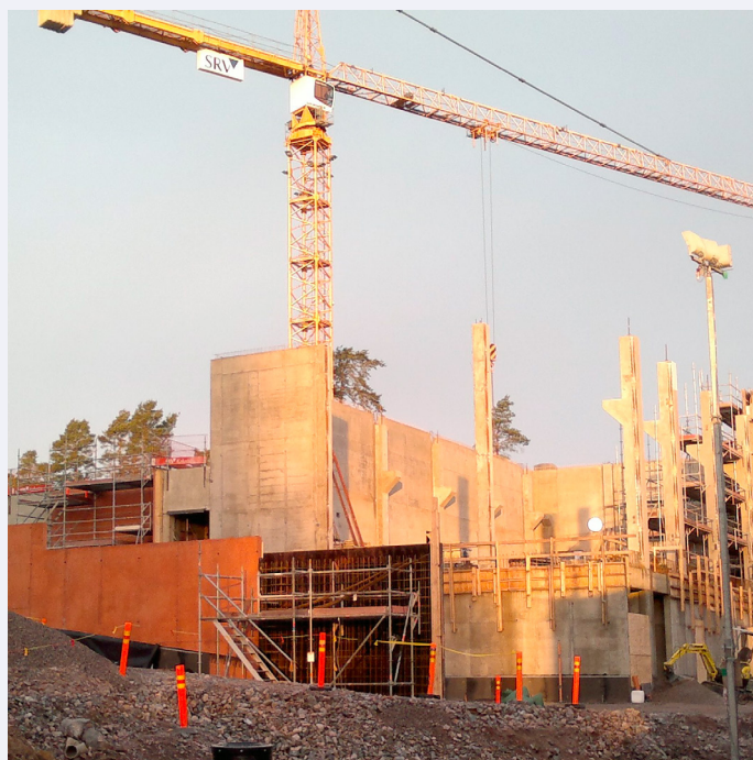
Figure 2. As the end of the first year of construction approached, the pillars and modular wall slabs were placed atop the 75 cm thick, pre-tensioned concrete floor of the main high-bay for the lead-shielded hot cells forming the heart of the facilities.
