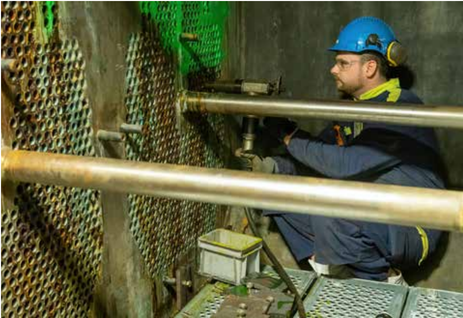
Dismantling of condenser tubes in one of the Oskarshamn units (photo: Uniper).
