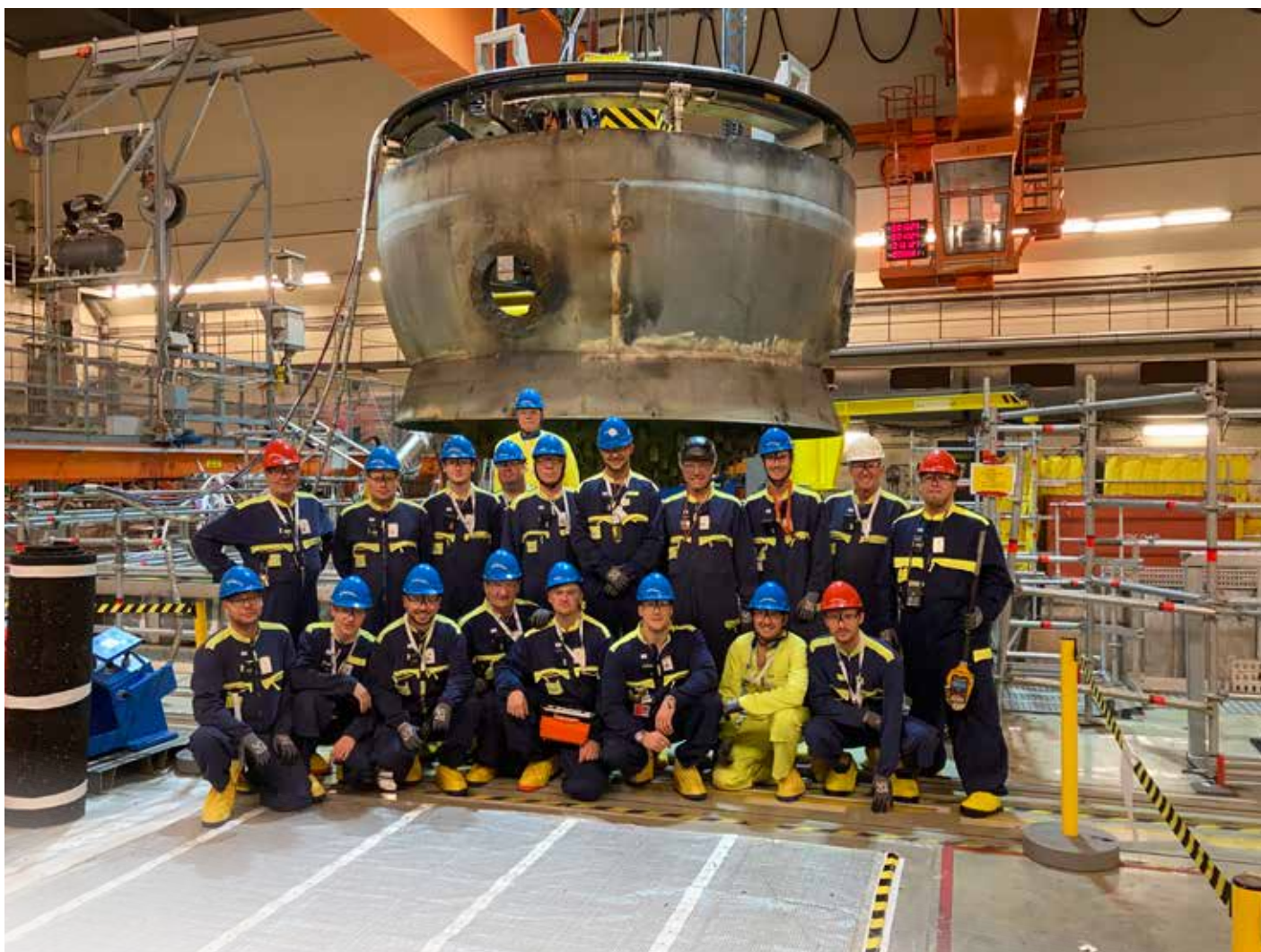
The first Reactor Pressure Vessel in the four-unit ND&D program to be completely removed from its original location. Now the Barsebäck 1 RPV is heading for final segmentation and waste management (photo: Uniper).
