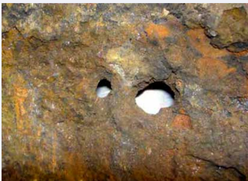
Figure 2. Corrosion damage in the steel liner detected at Ringhals-2 [7]. Complete penetration of the liner due to corrosion is visible.
